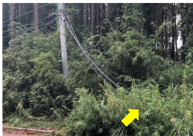
Fig. 1 Severed Power Lines Caused by Uprooted Trees
