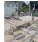
Wastewater treatment facilities
