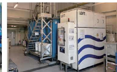
Liquid waste evaporation system
