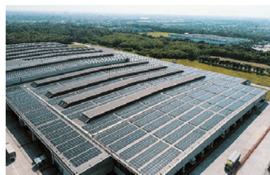
Solar panels installed at TMMIN
