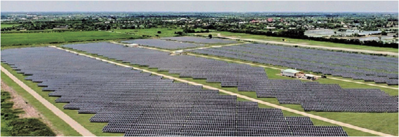
Solar farm of Toyota Motor Thailand Co., Ltd.
