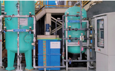
Wastewater recycling system
